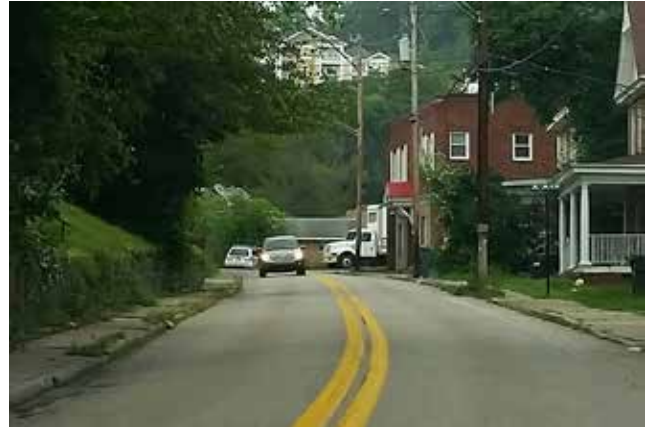
Sidewalks in need of repair on Willey Street in Morgantown
